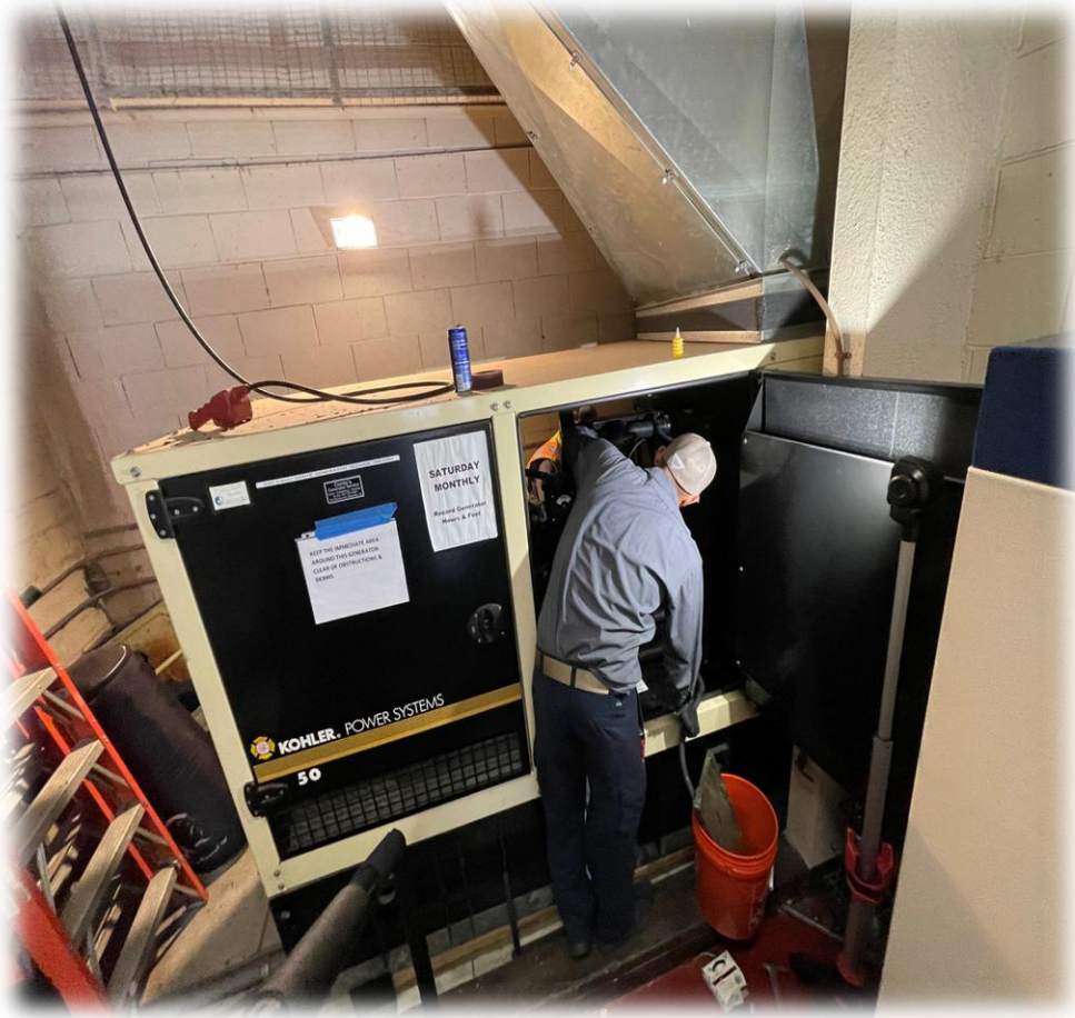
Fire Station Generator Inspection
